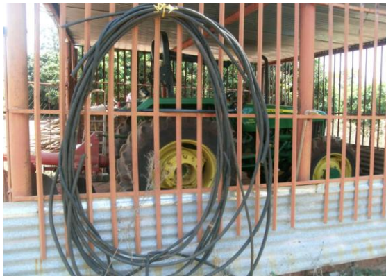
Figure 5 : Incomplete Irrigation system Installation
